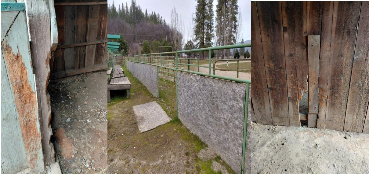
(left) damage to horse barn stall entry (center) bucking chutes standing area and fencing (right) damage inside stalls (Images courtesy of PCCGJ)
