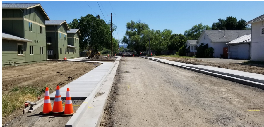
Orr Street development looking south toward Orr Street Bridge from the Orr Street/Brush Street intersection. (May 2020)
