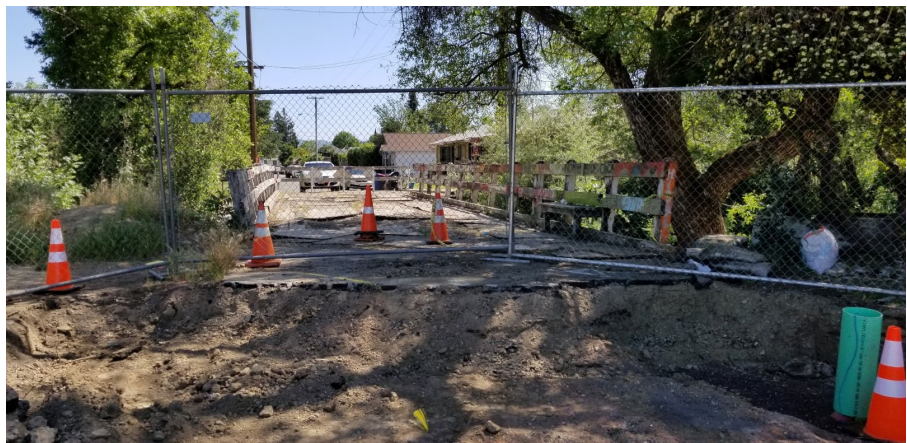
North side of Orr Street Bridge looking south into Wagenseller neighborhood with fence to prevent foot traffic entry into road construction from bridge. (May 2020)
