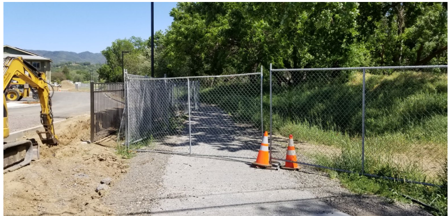
North side of Orr Street Bridge looking east along Orr Creek walking trail with fence to prevent foot traffic entry from trail to road construction. (May 2020)
