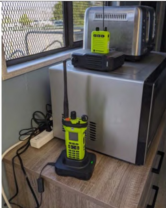
Alert system in modular trailer
