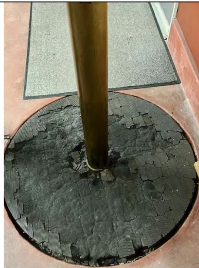
Poor condition of fire pole landing pad
