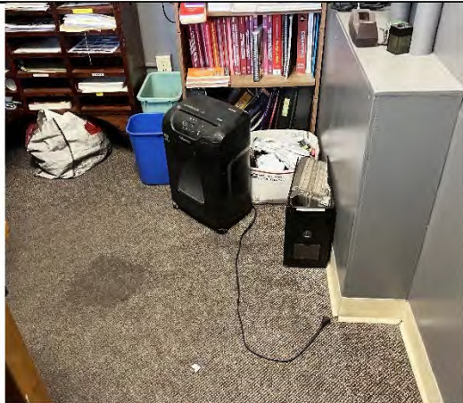
Worn out carpeting
