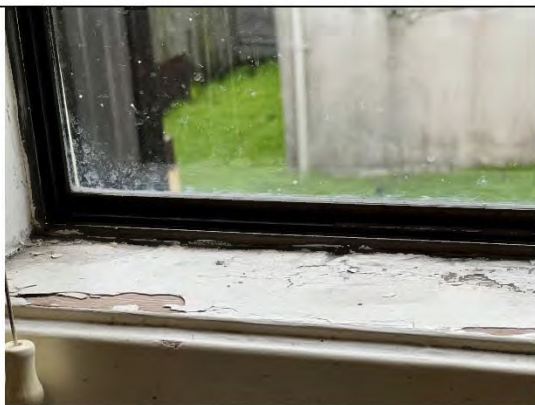
Window sill paint peeling
