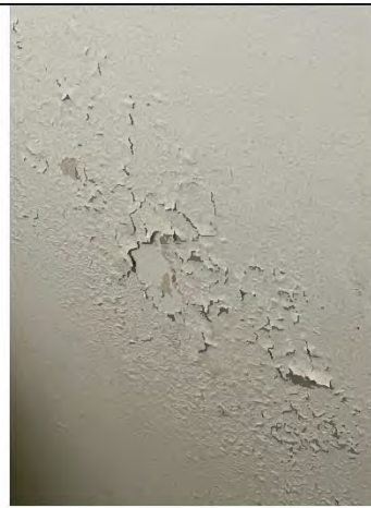
Kitchen paint flaking/peeling
