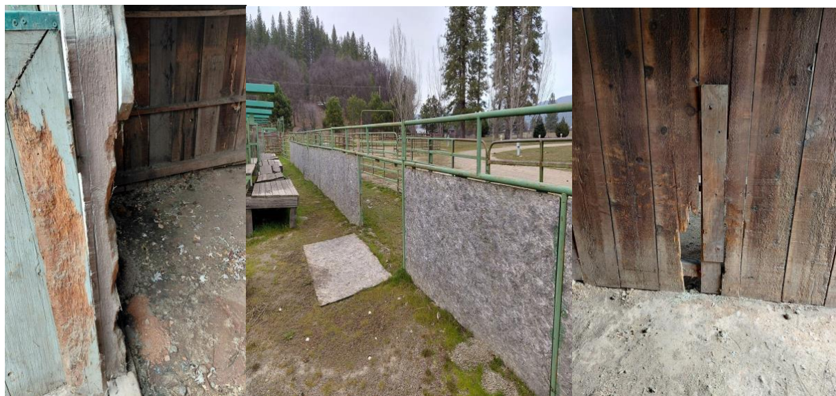
(left) damage to horse barn stall entry (center) bucking chutes standing area and fencing (right) damage inside stalls (Images courtesy of PCCGJ)
