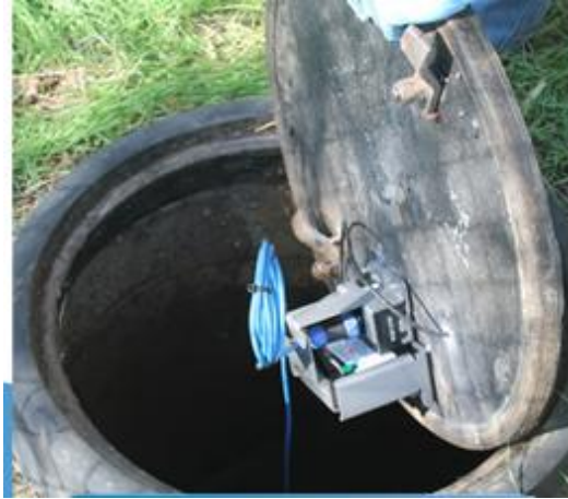
Flow meter to detect a breach in the sewer system Picture from Smartcoversystems.com
