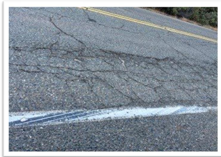
Alligator cracking on Wentworth Springs Rd. at Chipmunk Trail, Georgetown, July 2024
