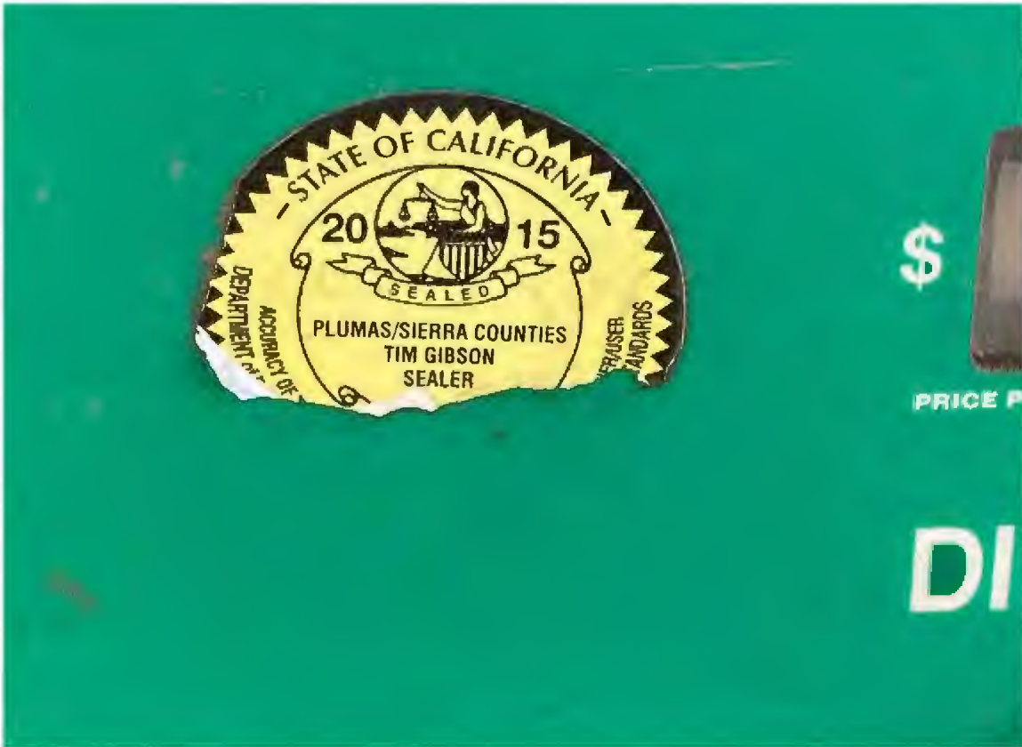
Figure 3 - Fuel pump last inspected in 2015 which is 4 years out of inspection compliance.
