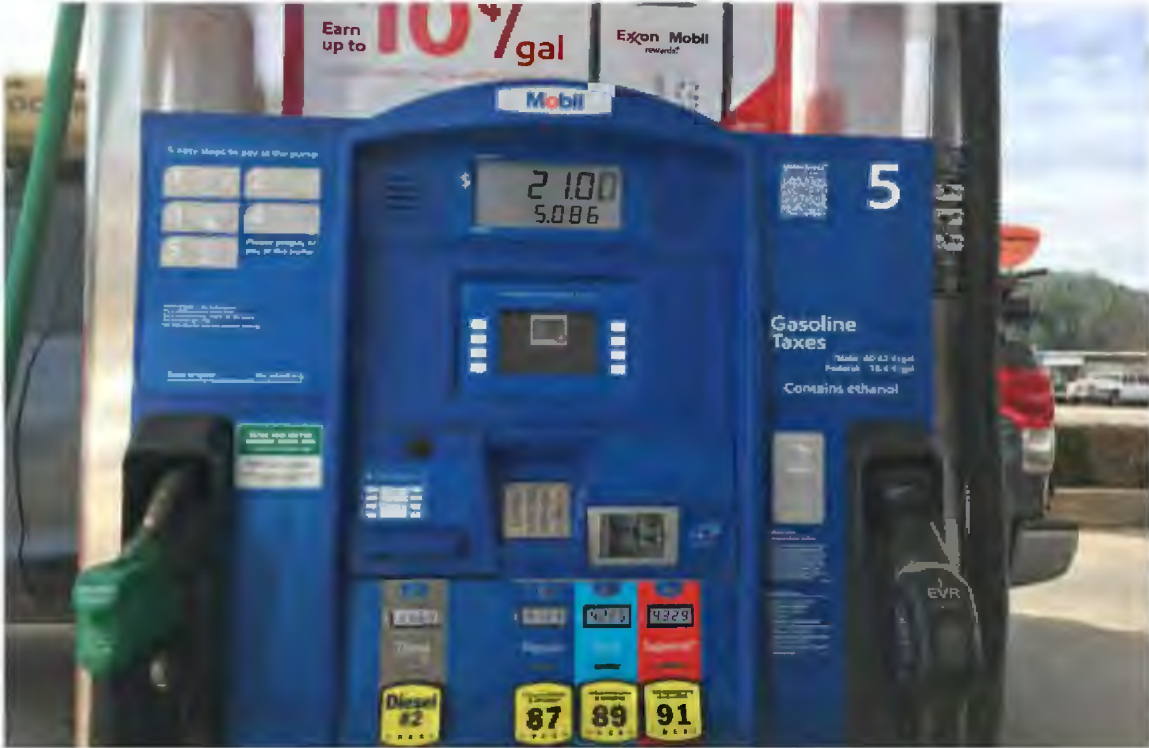
Figure 2 - Four fuel pumps (diesel and 3 grades of gasoline) with no yearly inspection sticker attached.
