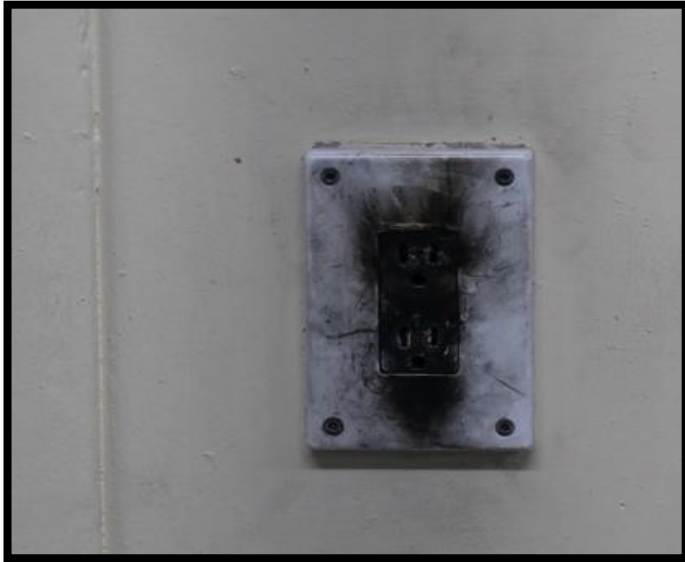
Damaged electrical outlet in housing unit
