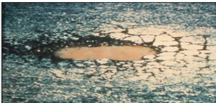
(Photo: LTPP Distress Identification Manual – DOT/FHWA)
