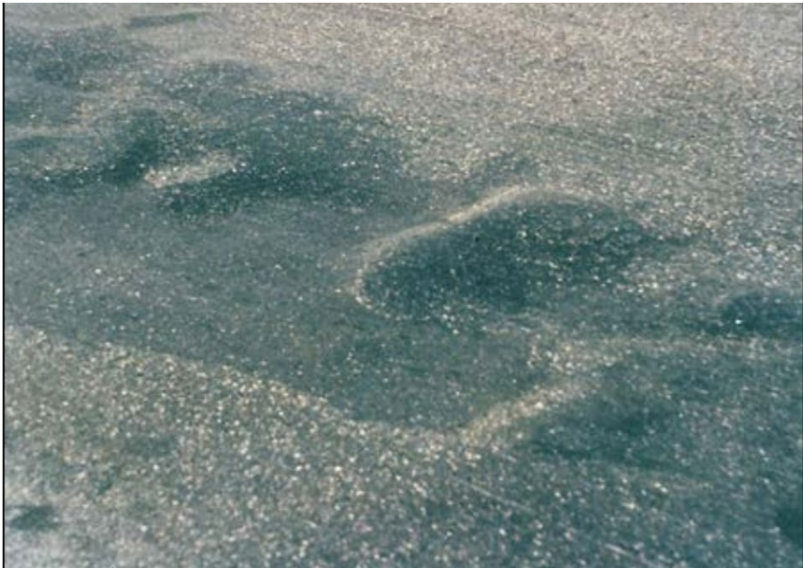
(Photo: LTPP Distress Identification Manual - DOT/FHWA)
