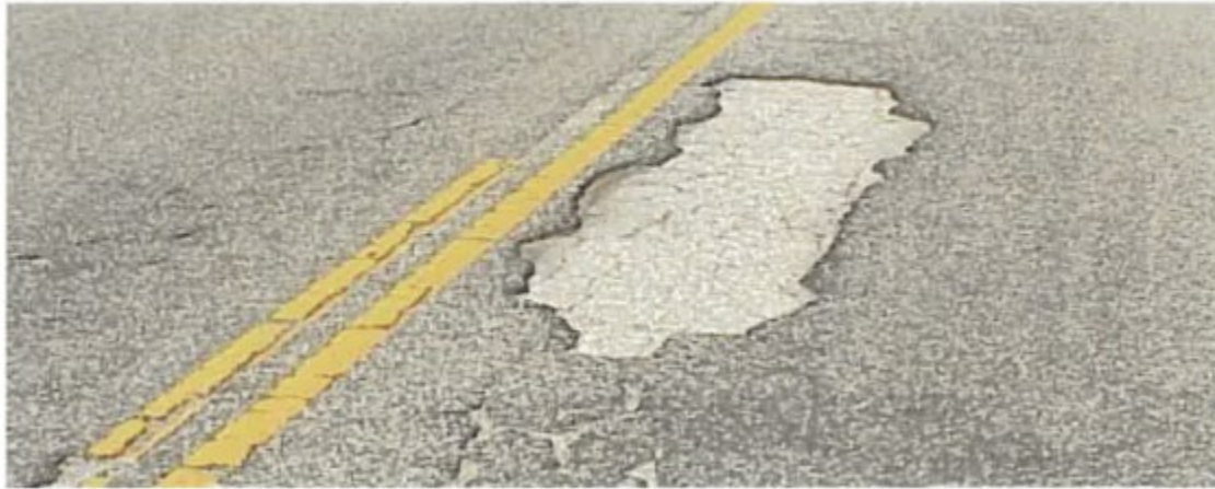
(Photo: LTPP Distress Identification Manual - DOT/FHWA)
