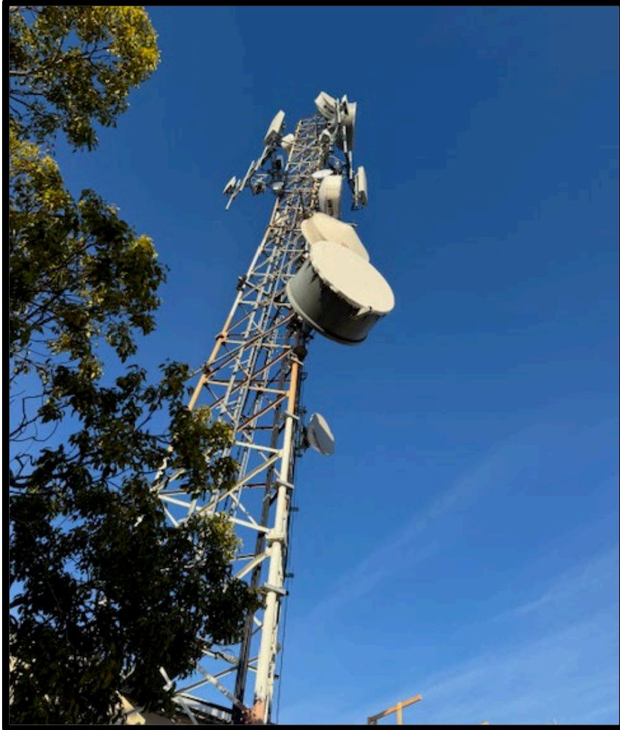
Tower in Salinas with various affixed communication Devices that are directed to the various communication towers throughout Monterey County
